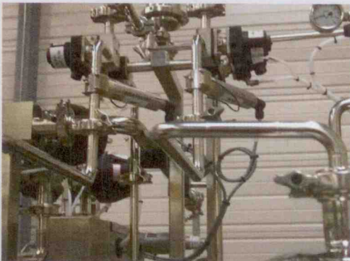
SONOCONTROL 15 installed within a pharmaceutical plant
